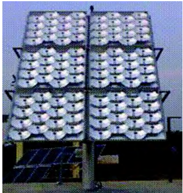
Fig. 12: A 1.2 kWp tracker set up by Moser Baer Photovoltaic Pvt. Ltd. Each of the parabolic mirrors has a high efficiency solar cell located at the focus. A similar tracker has been installed at IIT Kanpur by the company
