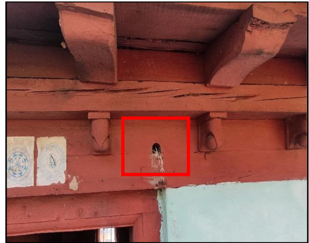
Fig. 15 A Pinjar can be seen in the red box. ICHR Project work
